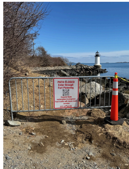
Pathway closed due to severe erosion
